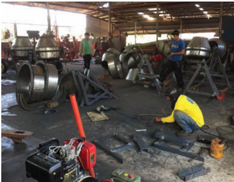
The project involved many facets, including building toilet facilities that would last and then hauling the parts to the villages for assembly.
